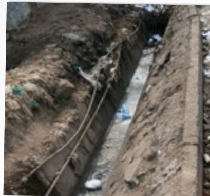
A SEWER RUNS THROUGH IT
